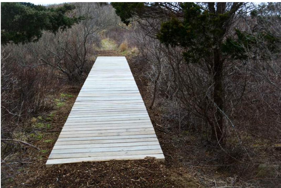
A new path between the lighthouse and the shops was installed in the fall of 2015 and includes a boardwalk. The path was installed with the goal of separating some of the pedestrian traffic from vehicular traffic
