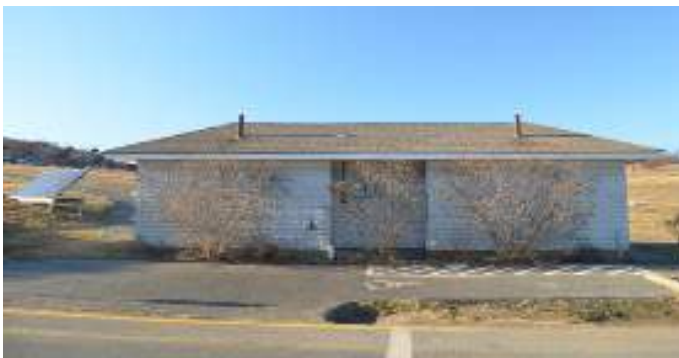
The bathrooms are out of place and highly visible. Maintenance is expensive and septic systems damage the surrounding ecology.
