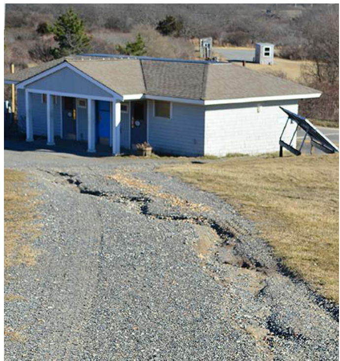
Heavy rains erode the uneven gravel path leading to the bathroom, more than 500 feet from the shops, lighthouse and overlook.
